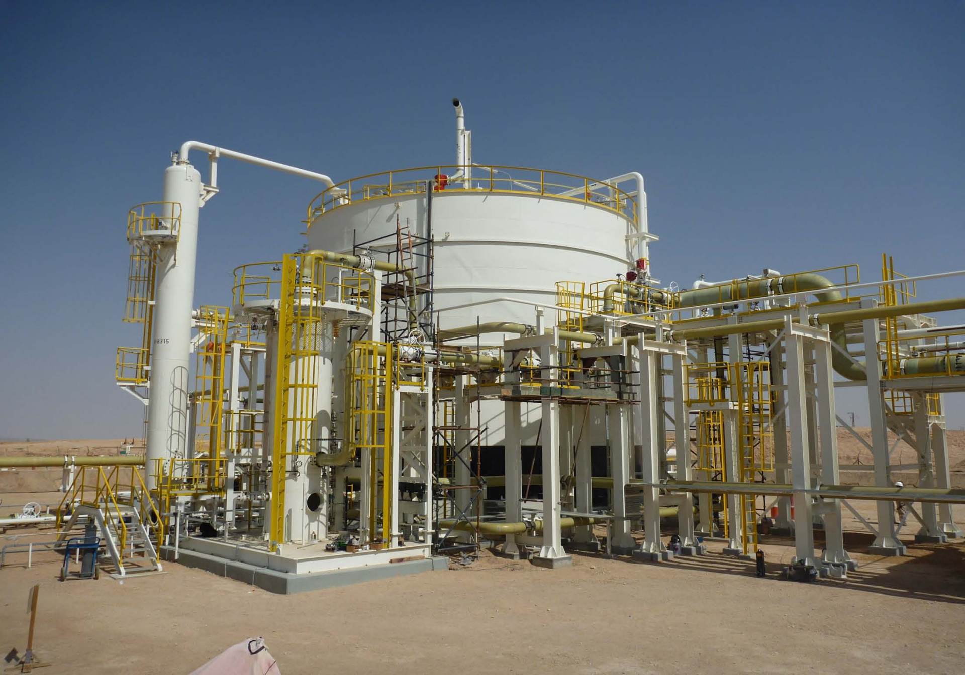
Figure A. Two Chamber GFT with GLR reactor Installation.
