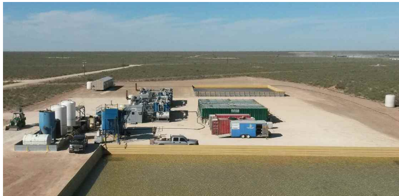
2 NOMAD Permian Facility (8,000 bpd feed capacity). Feed (PW) containment in foreground, heavy brine containment in background.
